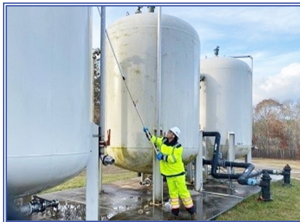
Carbon filtration vessels, maintenance and cleaning efforts
